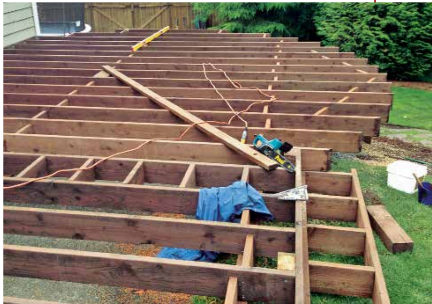
Figure 2. The author screws a beam compass—a length of 2-by or decking stock equal to the length of the radius—to the pivot point at the center of the circle and uses it to mark the circle's circumference on the joists.
