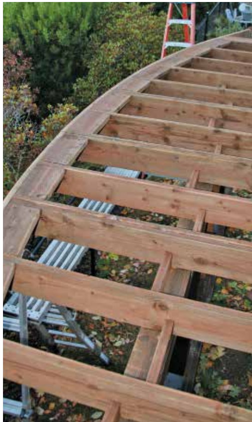
Figure 4. The author installs blocking at the ends of the joists to provide solid backing for decking fasteners.
